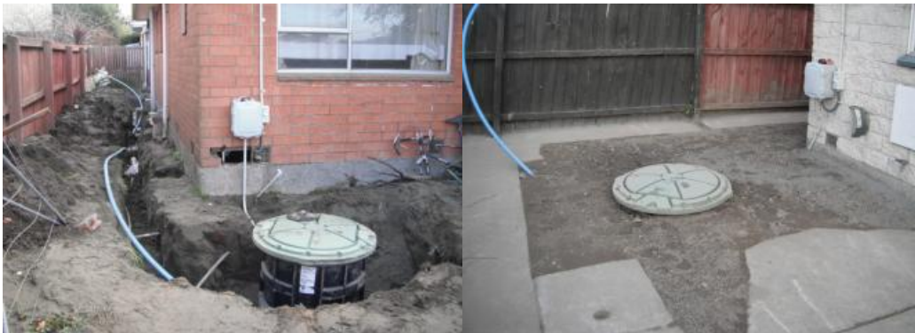
The installation of the pressure sewer systems in Avonside Drive and Ardrossan Street
